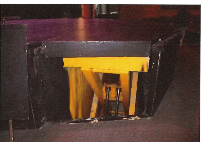
Lift at Upper Elevation
