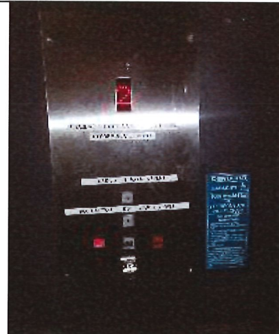
Car Operating Panel
