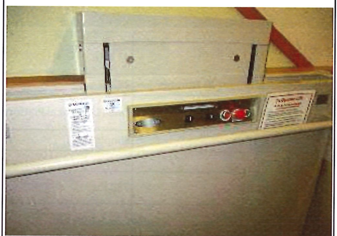
Car Operating Panel
