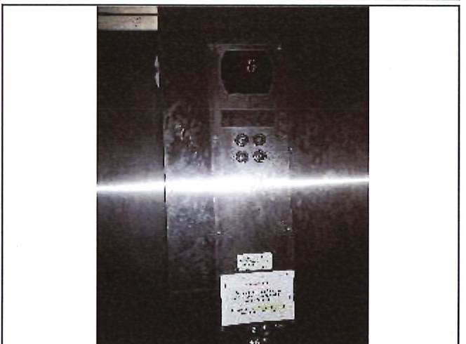
Car Operating Panel
